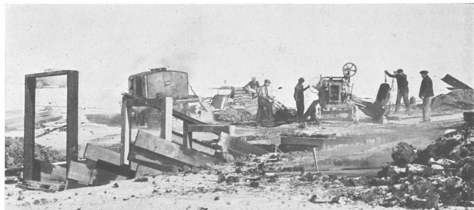
3 Foundations for the derrick are the next order of business. The forms have been completed and the concrete is being poured.
