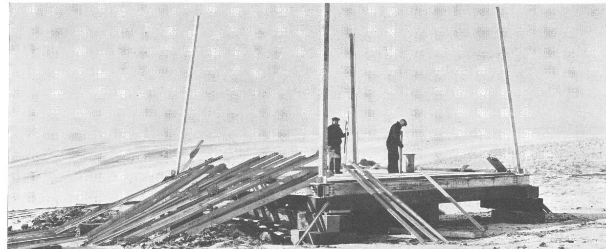
4 The derrick gets under way. The base is 30 feet square. The cost of such a derrick, unassembled, in the Turner Valley is approximately $7,800.
